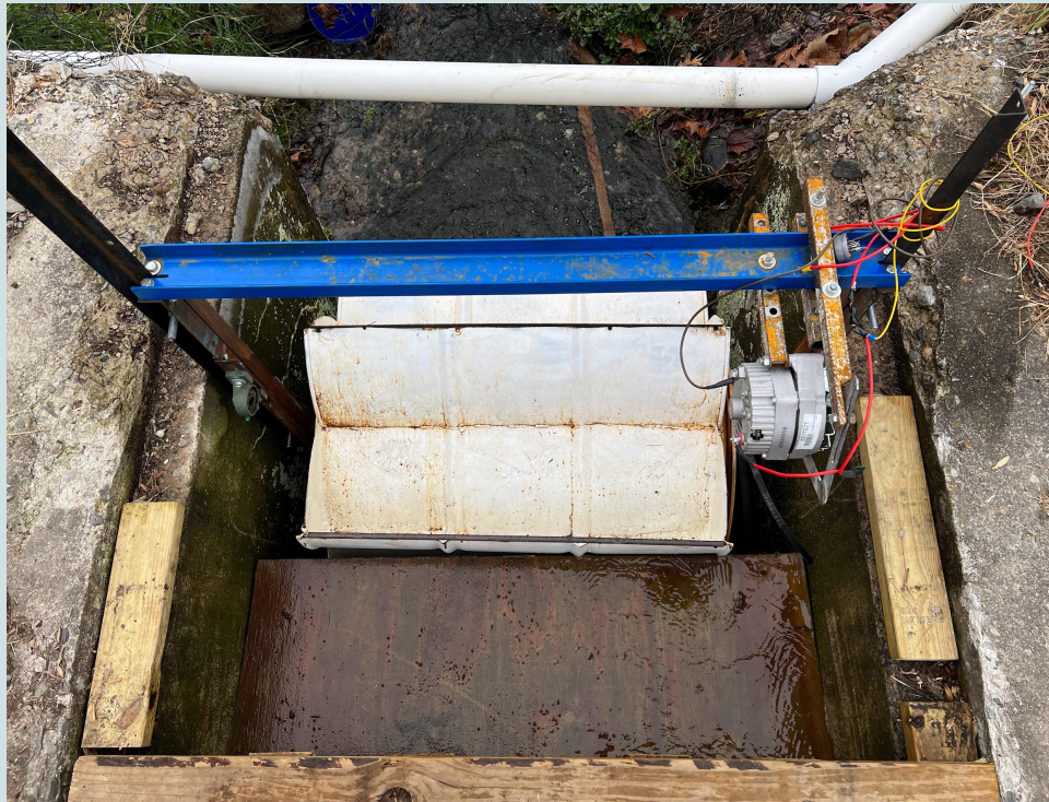
Water wheel before flood
